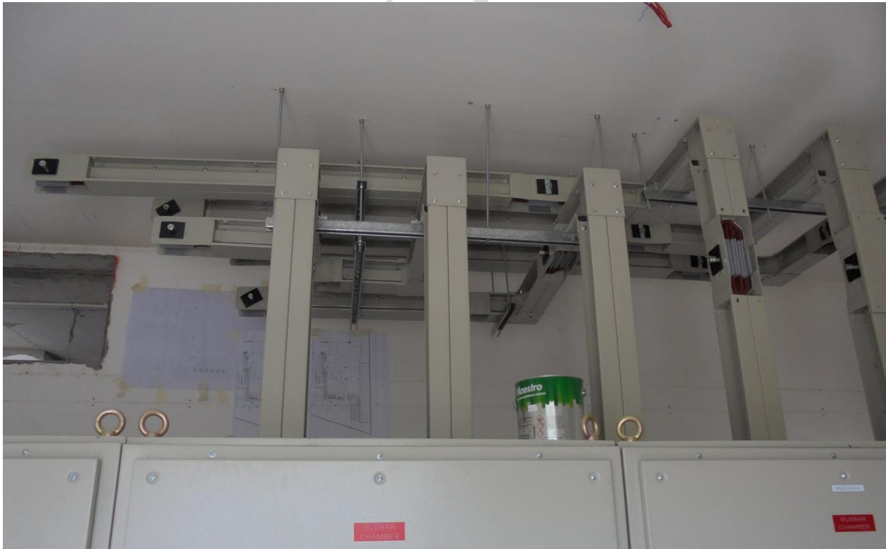
BUS BAR Riser & TOP OFF Unit
