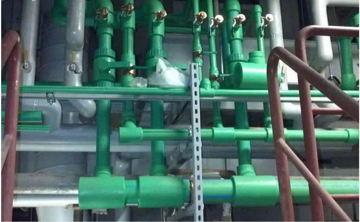
Pumping System for Supply Water
